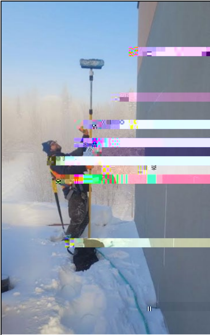
Ed Robinson from the HVAC shop had to climb out on the roof of Lathrop this past weekend to clear the ice buildup from the air intake. Nice job with the safety harness! Thanks to Thadd Williamson for the photo.
